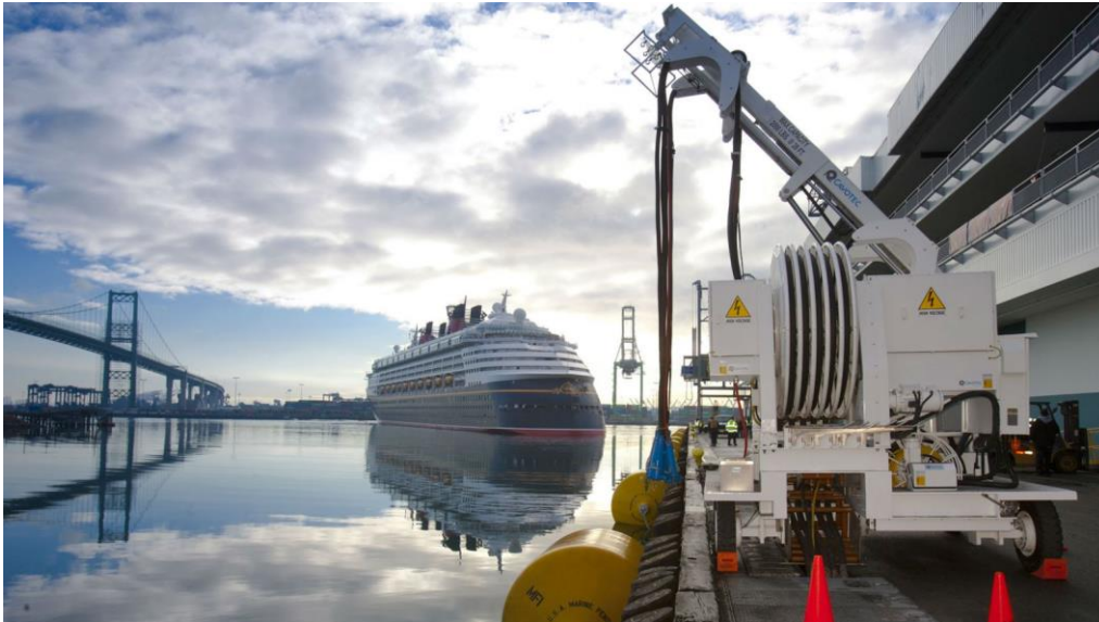
Figure 11 Shore power at the Port of Los Angeles
